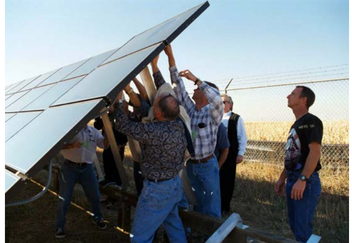
Photo by Western Area Power Administration, NREL 08822
