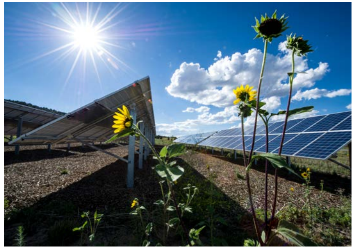
Photo by Dennis Schroeder, NREL 26962
